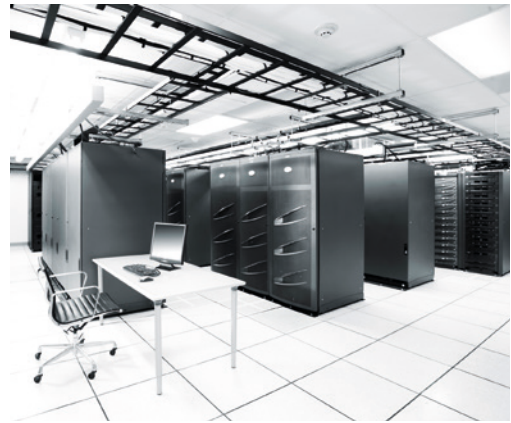
Fig. 116: Typical CRAC devices.
