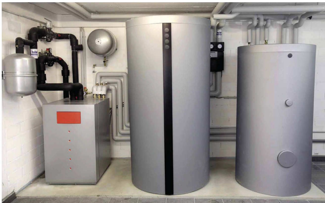
Fig. 121: Heat pump with potable hot water storage tank.
