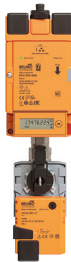
Fig. 49: An Energy Valve that does not meet its flow requirements and has insufficient differential pressure.
