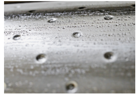
Fig. 93: Condensation of humid air on the cold coil surface. The supplied cold water must be above the dew point in the room to prevent condensation.
