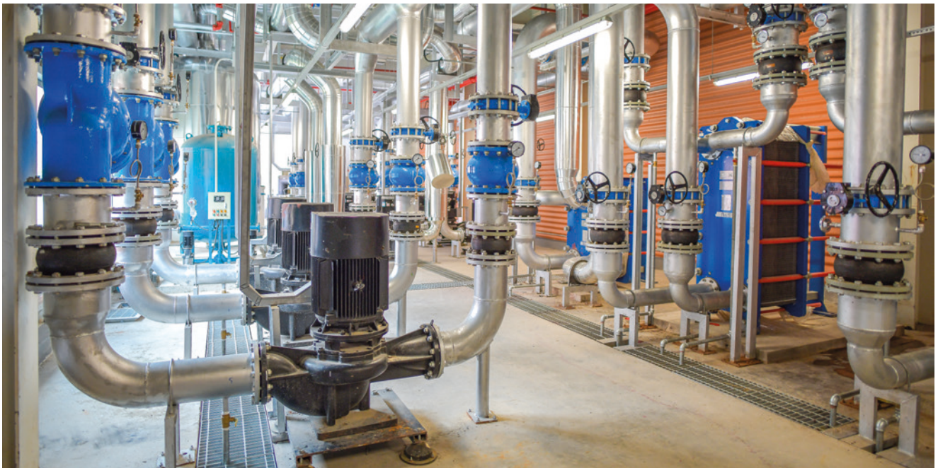
Fig. 67: Heat exchange station
