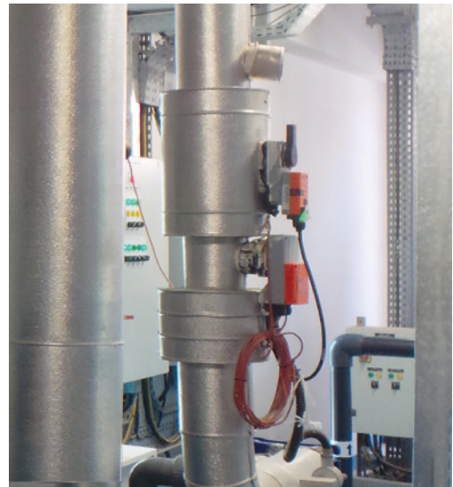
Fig. 89: The supply of the fan coils is equipped with the Belimo Energy Valve™.
