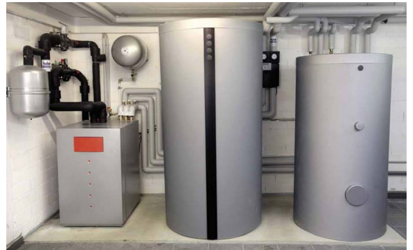
Abb. 114: Heat pump with potable hot water storage tank.
