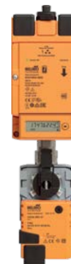
Abb. 42: An Energy Valve that does not meet its flow requirements and has insufficient differential pressure.
