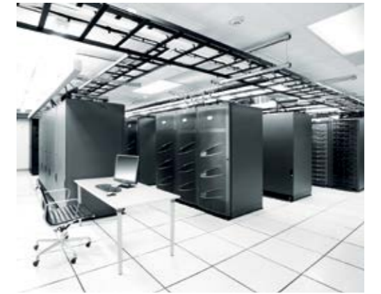
Abb. 109: Typical CRAC devices.
